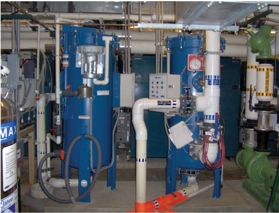
JW Marriott Filter Room showing Neptune-Benson's Defender Filters.
